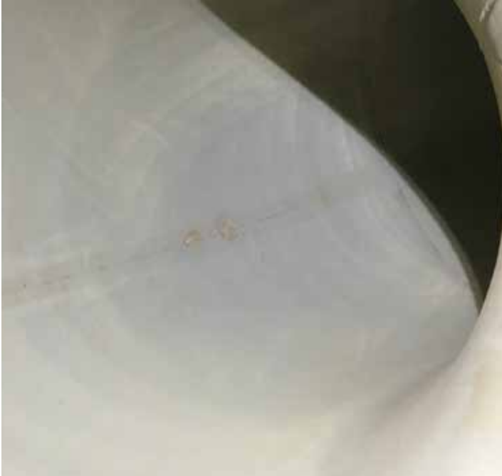
CONDENSER LINE AFTER 1 YEAR CHEMLINE® SERVICE
