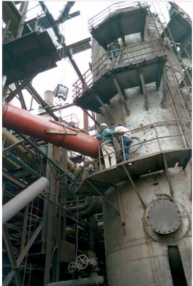
(Above) Installing pipe lined with ChemLine® coating to the scrubber, which is also lined with ChemLine® coating. (Left) Pipe section leading into scrubber lined with reinforced ChemLine® coating.
